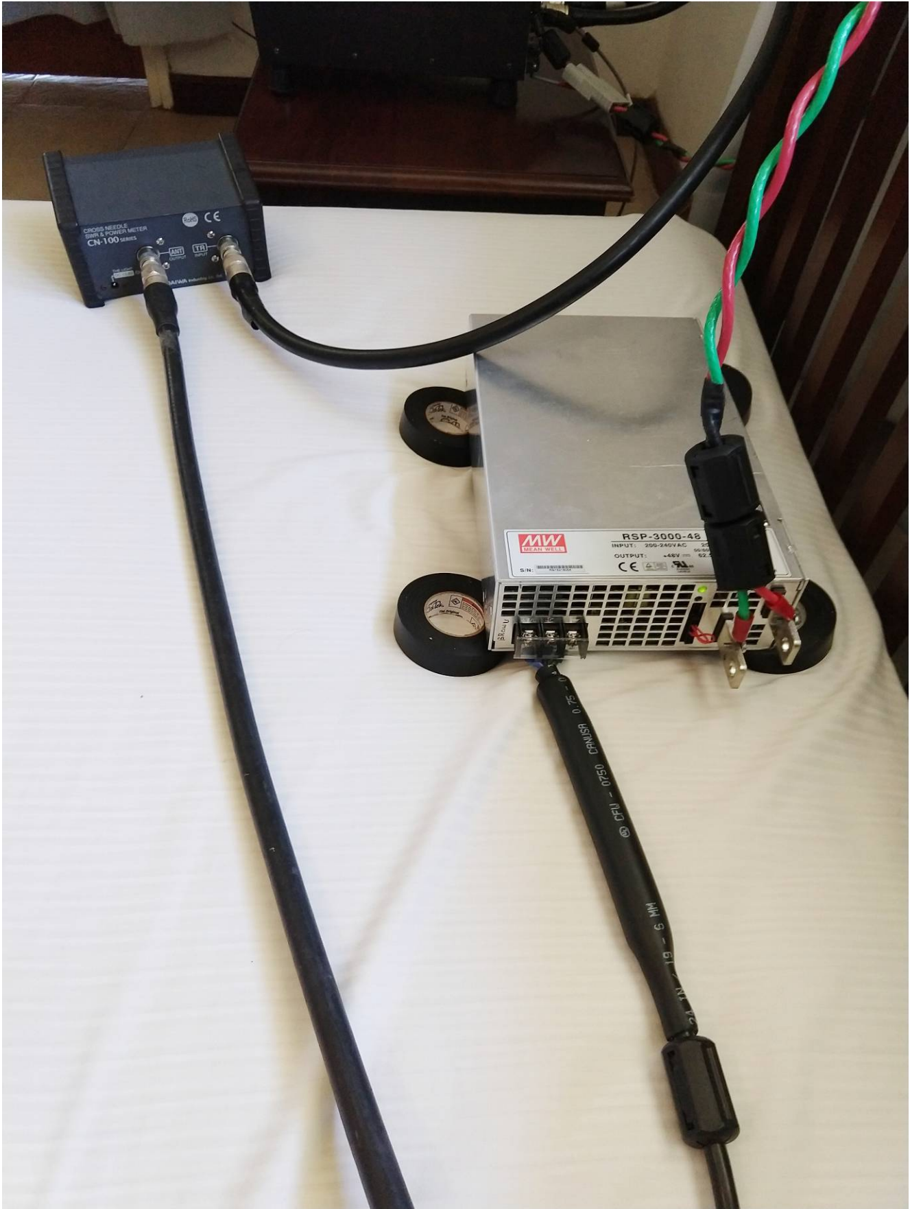
Note the multiple ferrite cores (covered with heat shrink tubing) and snap on ferrite filter on the AC input to the Meanwell RSP-3000-48, and the snap on ferrite filters on the DC output and again at the DC connection to the amplifier.
